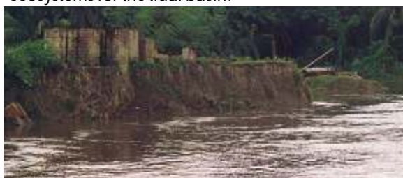
Erosion along the left bank of the Hari River at Solgati
