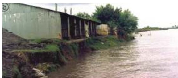
Erosion threatening the houses constructed for landless people under 'Asrayan Prokalpa' at the right bank of the Hari River near Solgati
